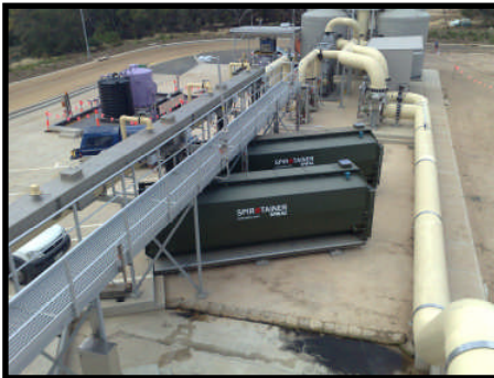
Sludge system with weigh scales and retractable chutes
